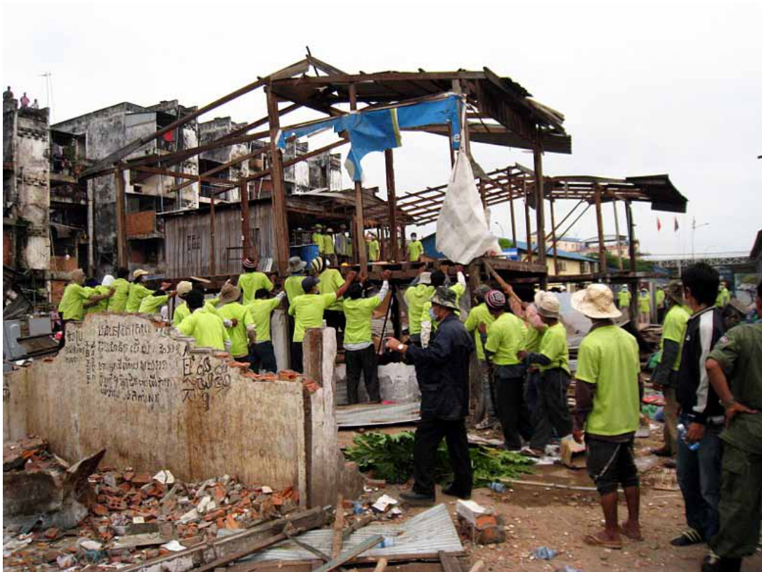
A line of workers push at the skeleton of a destroyed house, trying to topple it over.
