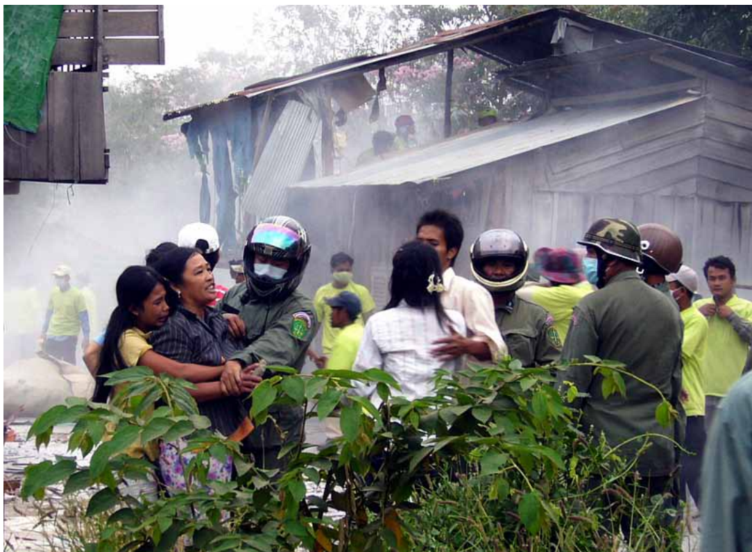
Police move residents away as demolition workers (in green) continue their work.
