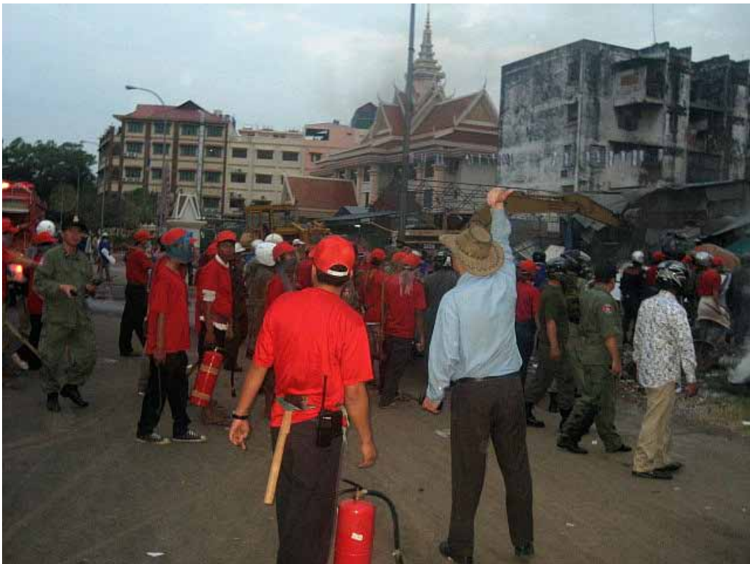
A 7NG company worker (in hat) signals for hundreds of demolition workers with machinery and tools to move in to start demolishing villagers' homes.
